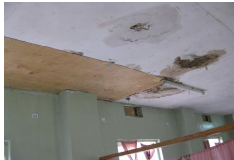
Buildings in disrepair
